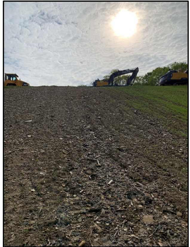
Photo 2 – Unstabilized Portion of Fill/Slope
